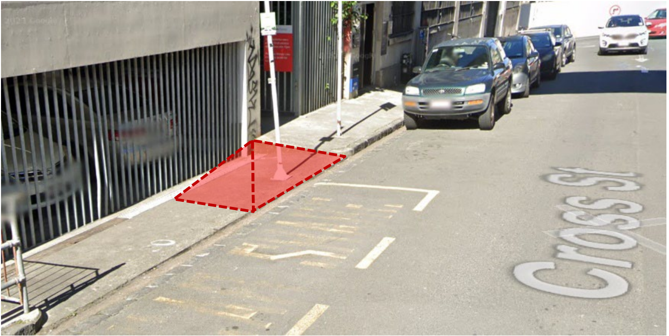
Figure 26: Existing abandoned vehicle crossing and uneven footpath step.
